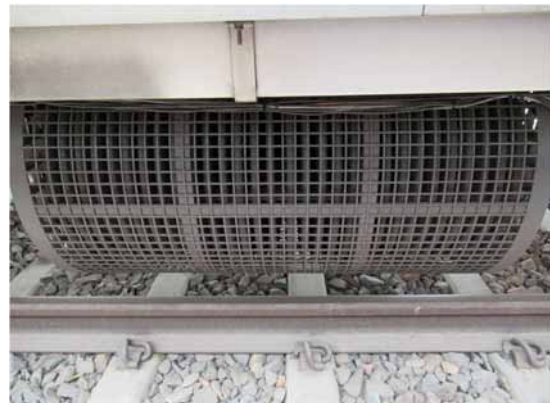
Fig. 8 Condition of cooler after one year of operation on the RS13 train (India Delhi metro)
