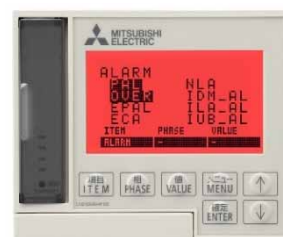
Fig. 5 Red backlight indication at alarm occurrence
