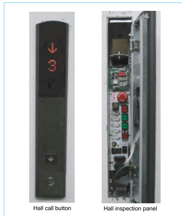
Fig. 6 Hall inspection panel behind hall call button
