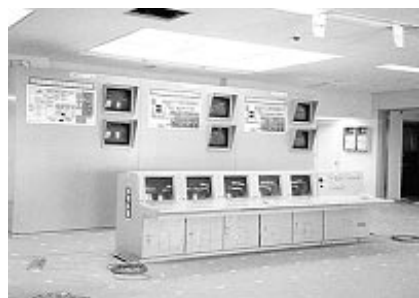
Fig. 4 Operator's station in the central control room.
